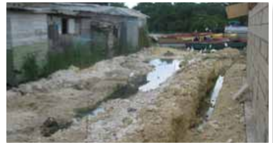
BEFORE: The drainage at the Black River Fishing Beach was unstructured and prone to erosion.
