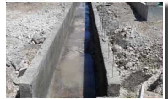
AFTER: The construction of a new concrete culvert will increase carrying capacity of the drain and prevent further erosion.
