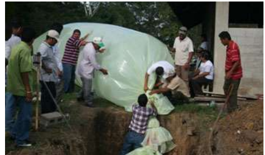
Eight biodigesters were installed in three districts of Belize.
